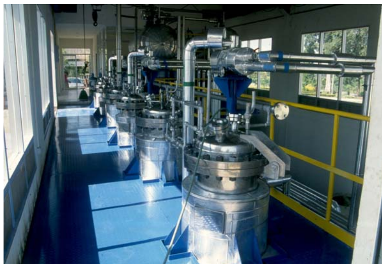
Commercial HFC-134a based extraction facility, Phurua Natural Oils Ltd, Thailand. (Courtesy of Peter Wilde Associates Ltd).
